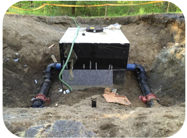
Master Meter Vault at Water Treatment Plant
