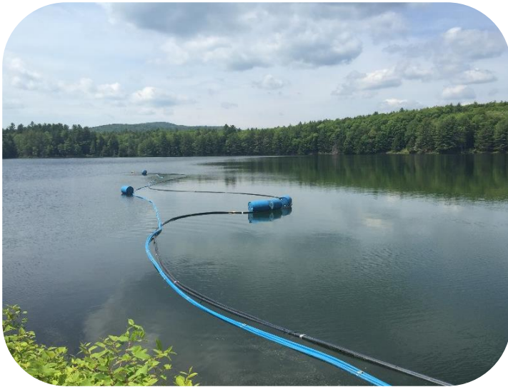
Chemical Feed, Level Sensing, Raw Water Sampling Tubing to the Raw Water Intake on Minard's Pond (prior to sinking)
