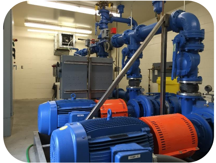
Interior View of the Commonwealth Pump Station
