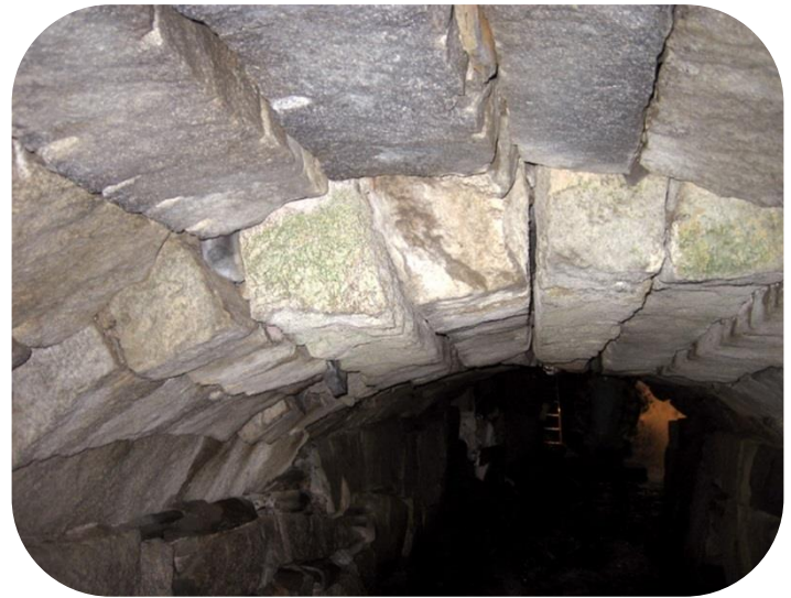
Failing arch culvert
