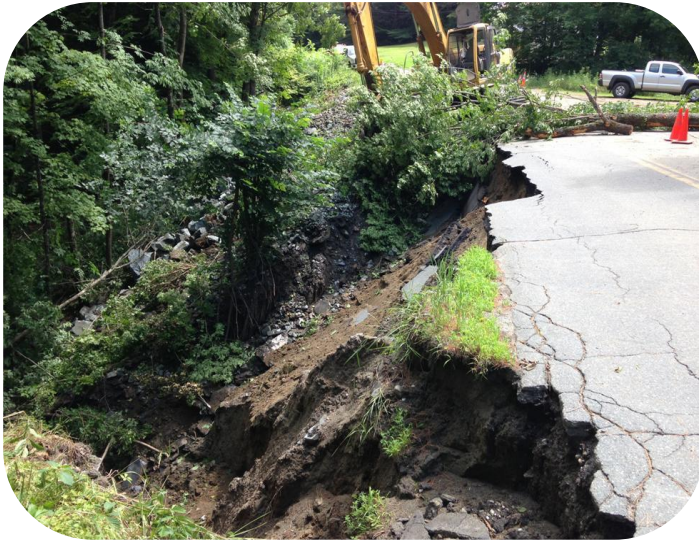
Slope failure after storm event
