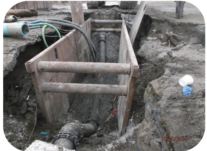
Water Main Relocation Required for New Utilities
