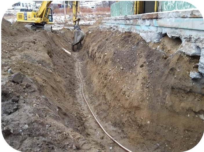
New service lines were left in front of existing buildings for future connections
